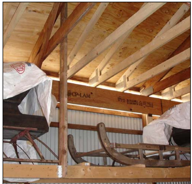
As part of the renovations to Bay #3 last winter, shelving was installed to accommodate several more vehicles. Patti Mikkelsen photo
